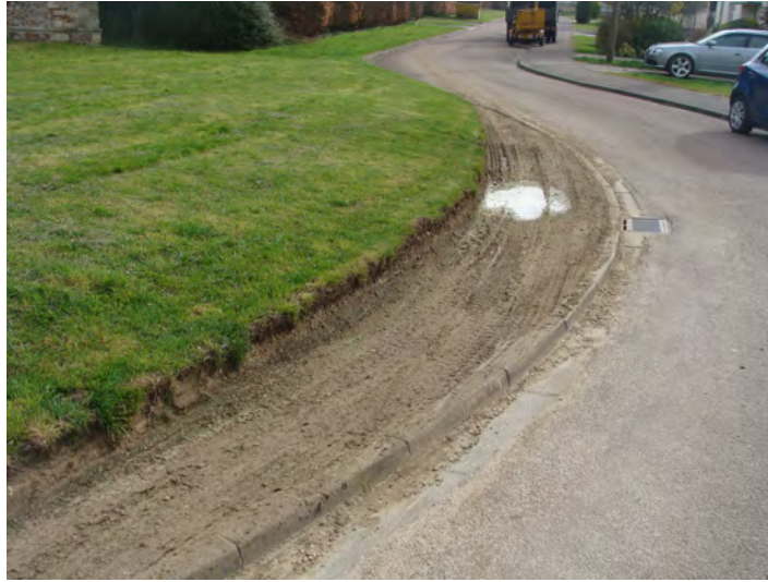
Picture 1.18 Badly eroded edge to open space fronting south elevation of church. A sensitive resolution of this problem would be beneficial
