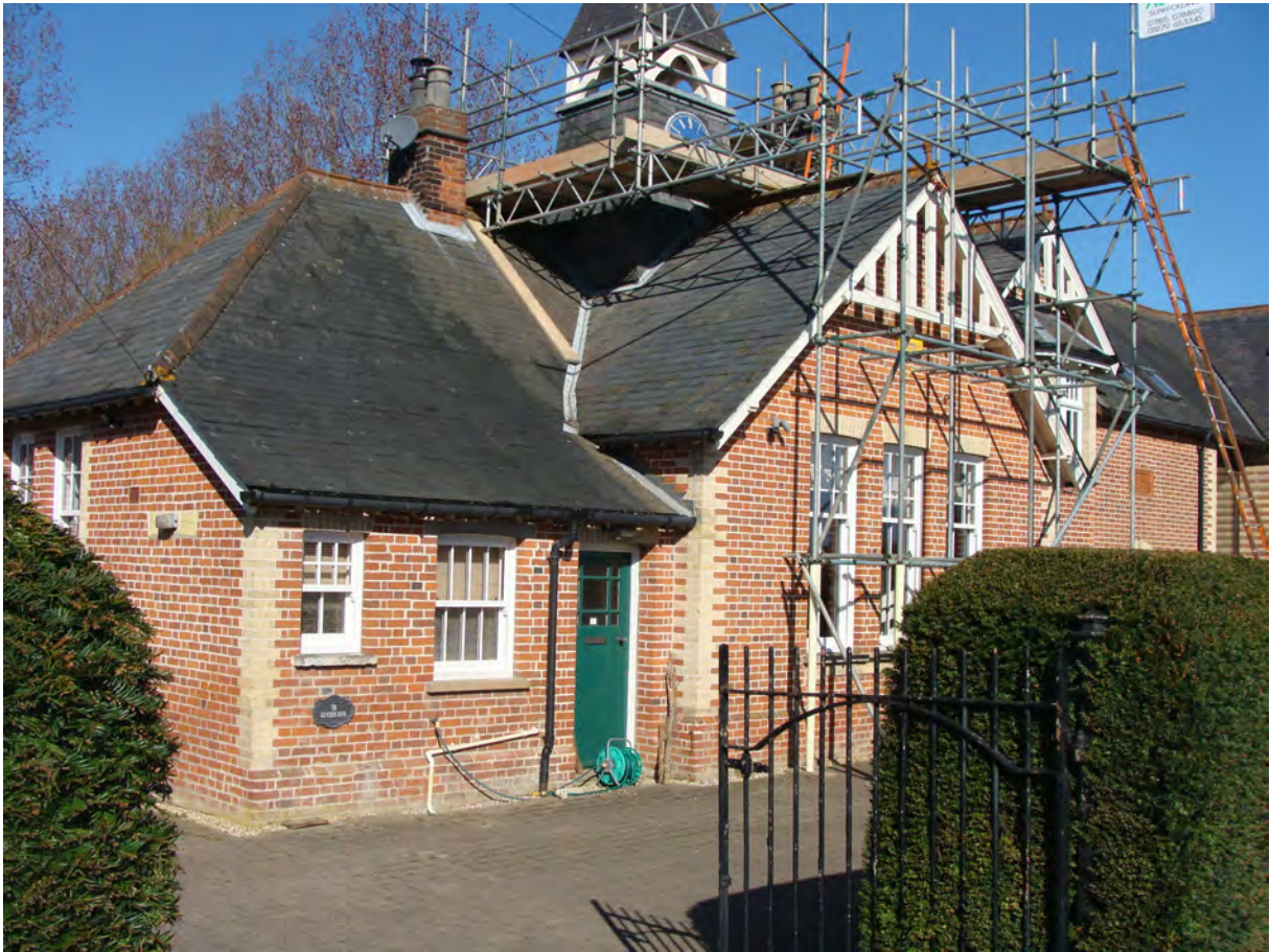
Picture 1.16 Old School House. A prominent and distinctive property at the northern extremity of the Conservation Area whose massing and architectural qualities provide a fine introduction to the Conservation Area
